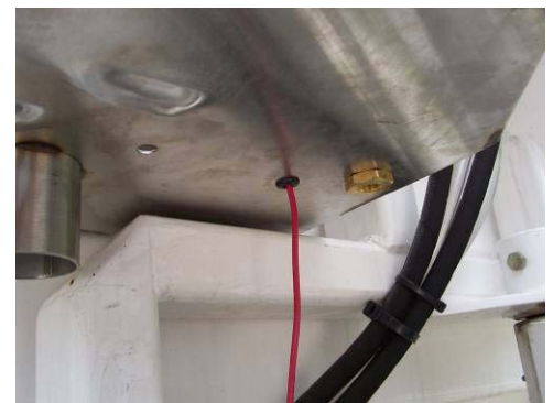
One can see the bolt that fixes the faucet and the wire which goes to the control panel.
