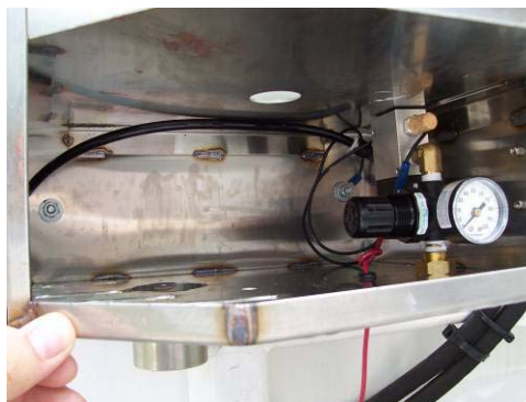
Connect one wire to the box (ground) and the other to a long wire which goes to the control panel. Make a node before the box hole to prevent pulling out this wire.
